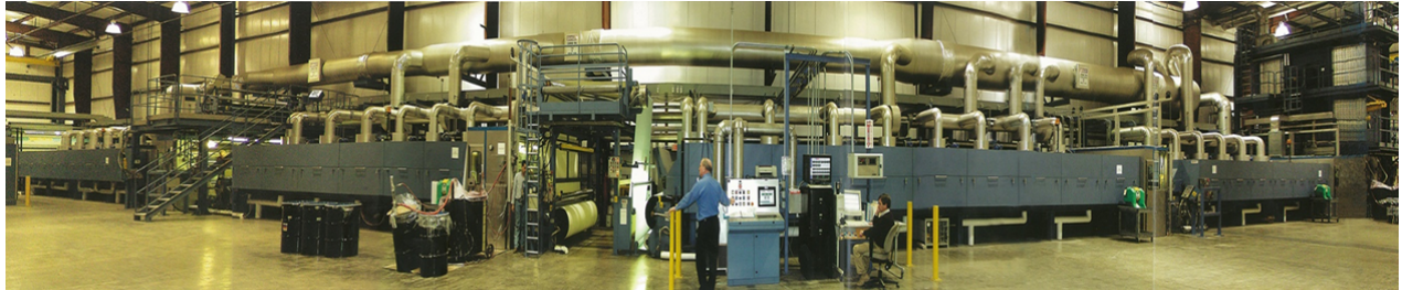
Figure 14 111m long foam coating and curing oven
